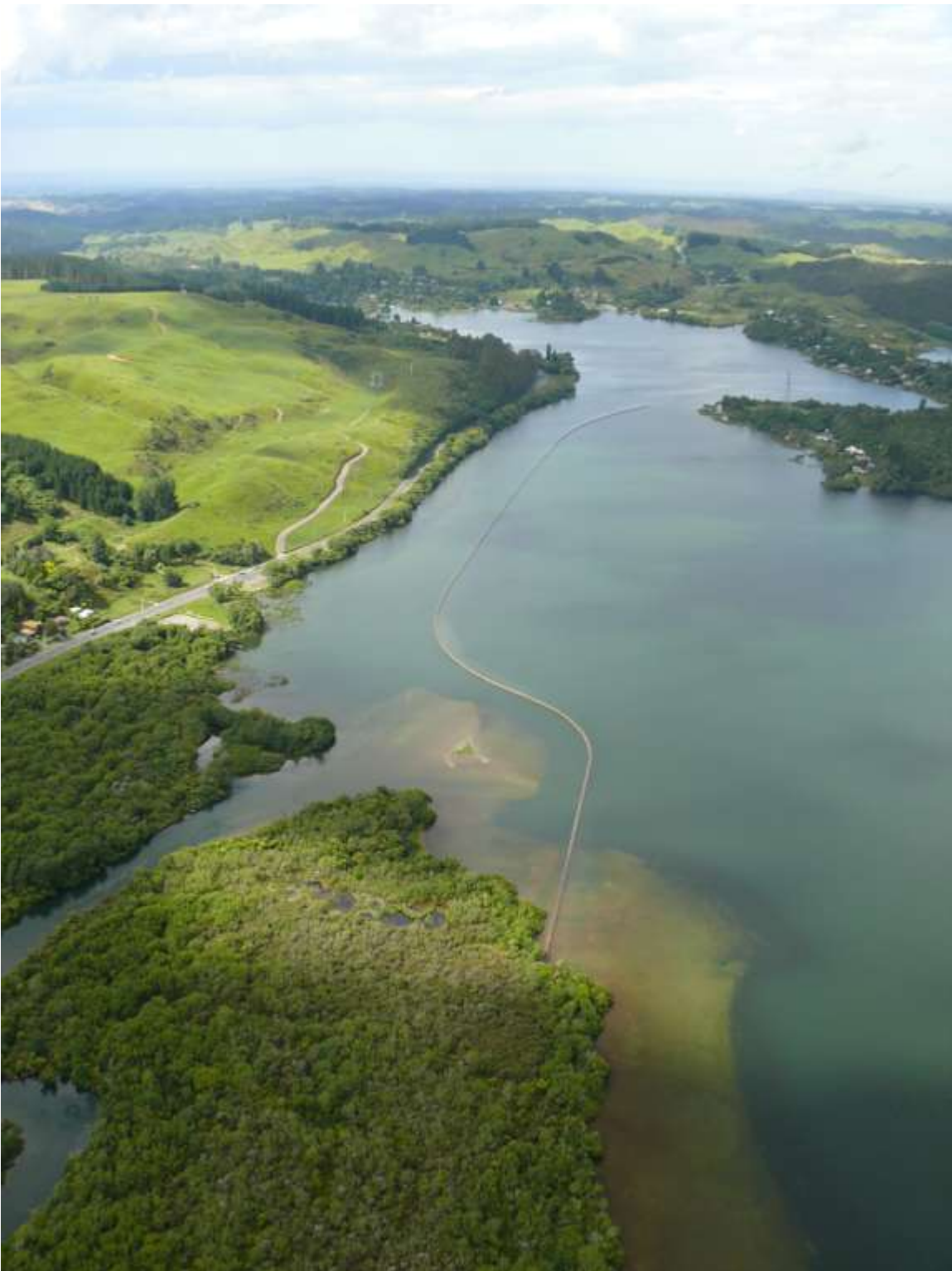
Figure 10. Photo of the Ohau Channel diversion wall showing the Okere Arm towards the outlet of Lake Rotoiti (upper left). Photo: Environment Bay of Plenty.
