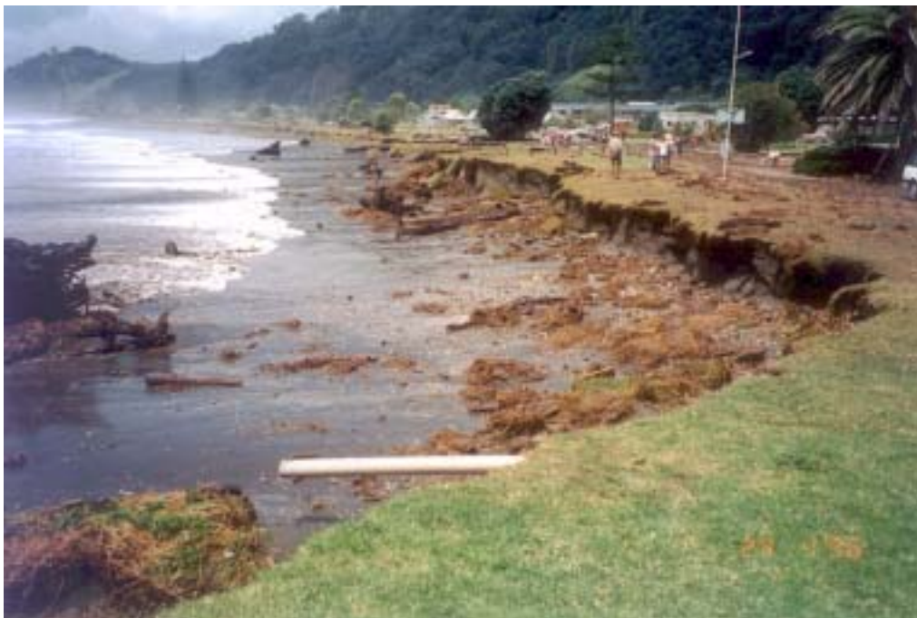
The western end of Ohope Beach in the 1996 storm shows the degree of erosion
